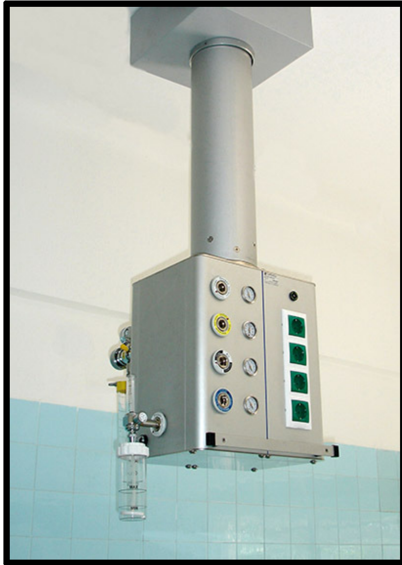
CENTRAL PIPELINE OUTLET AT O.T- PENDANT SYSTEM
